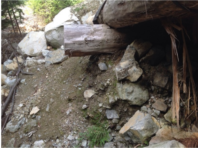
right downstream abutment scour
