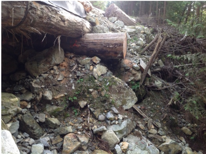
left downstream scour
